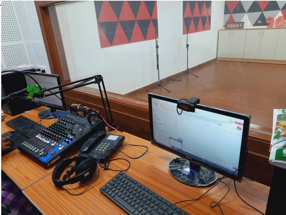
FM Broadcasting Equipments
